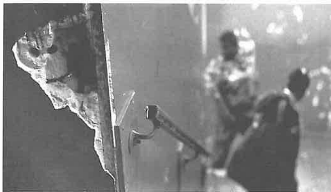
Under court order, walls like this one at Laundale Academy were repaired last year to halt lead exposure.
